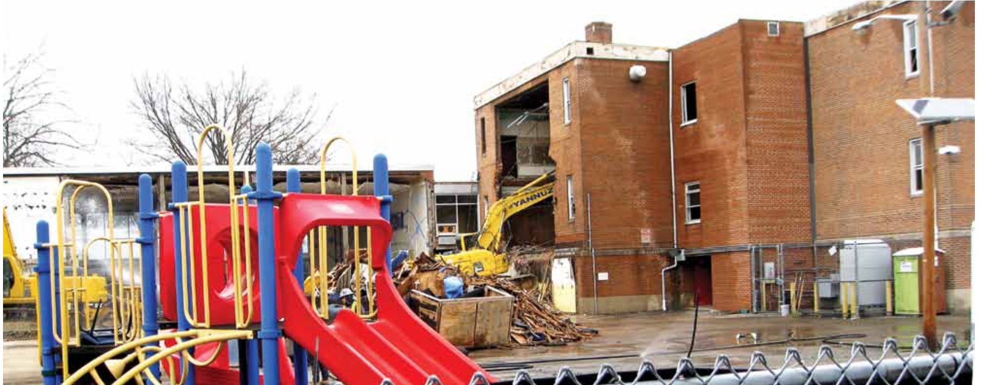
The BOE awarded a bid in August for $595,000 out of the district's capital reserve fund for the demolition, which was not part of the $38 million referendum. During the demolition, a time capsule from 1914 was found in the cornerstone. No one knew it was there. It will be opened March 3, 2024 at 3 p.m. in the Memorial School Gym.
